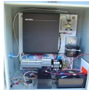
Telemetry equipment providing 24/7 monitoring of critical systems.
