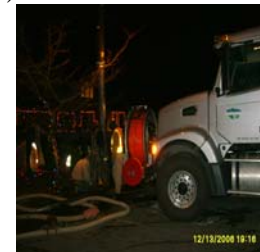
The District responding after hours water line break.
