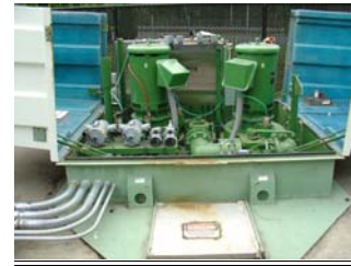
A wet well mounted lift station pump being serviced by District staff.
